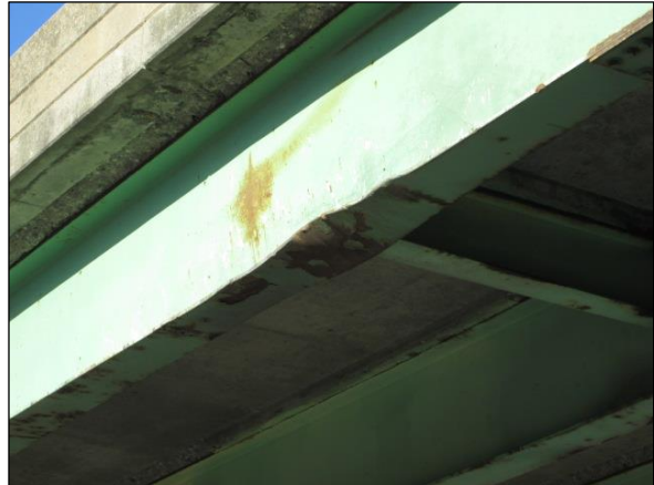
Bridge concerns include evidence that trucks have struck the bridges multiple times.
