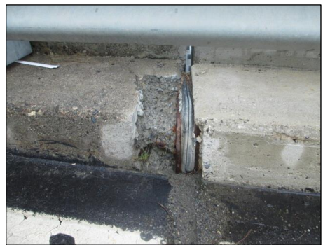
The two photos show concrete spalling and cracking, including a large section of concrete deteriorating from a bridge shoulder.
